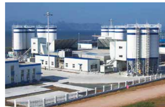
海阳核电2HZS150VG (核电站) 2HZS150VG (mixing plant for nuclear power plant construction) in Haiyang Nuclear Power Plant
